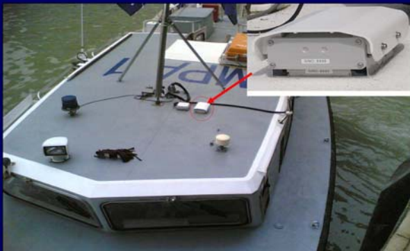
A TYPICAL INSTALLATION OF FIXED HARTS TRANSPONDER ONBOARD HARBOUR CRAFT
