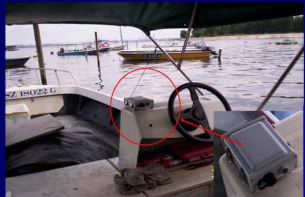
A TYPICAL INSTALLATION OF PORTABLE HARTS TRANSPONDER ONBOARD HARBOUR CRAFT
