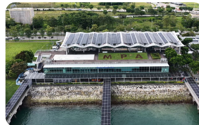
Solar photovoltaic panels at Marina South Pier
