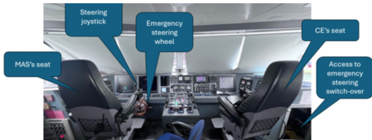
Fig. 7: Location of the emergency steering changeover switch on the bridge.
