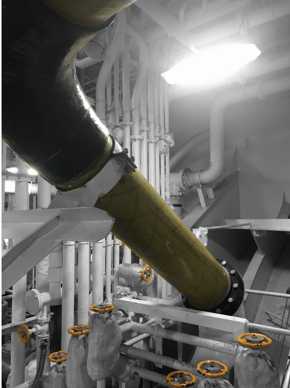
GRE pipe to overboard discharge.
