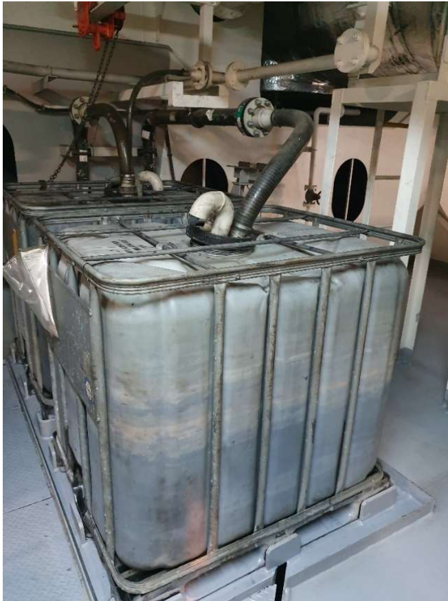
IBC tanks used for storing scrubber residue
