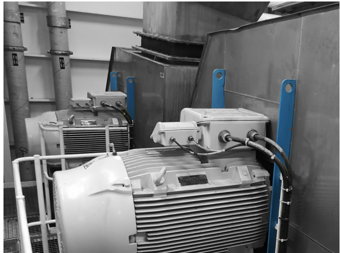
Exhaust gas extractor fans to reduce backpressure
