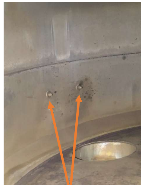
High level sensors
