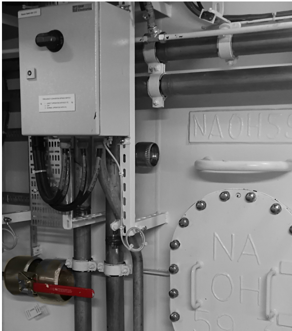
Caustic soda storage tank onboard a ship.
