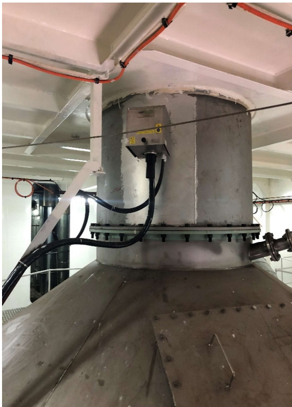
Top of scrubber tower and deckhead, without any fire detectors nor fixed fire-extinguishing arrangement
