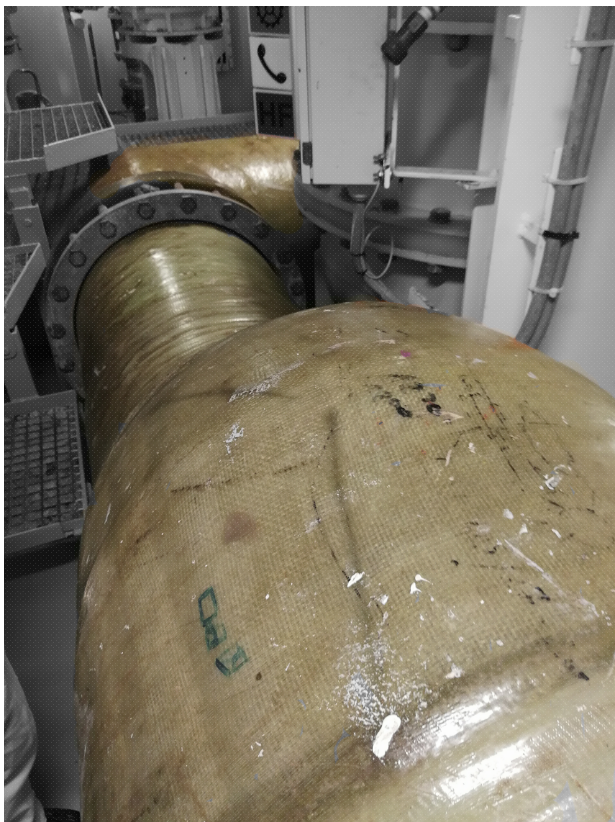
Close up view of a GRE pipe section
