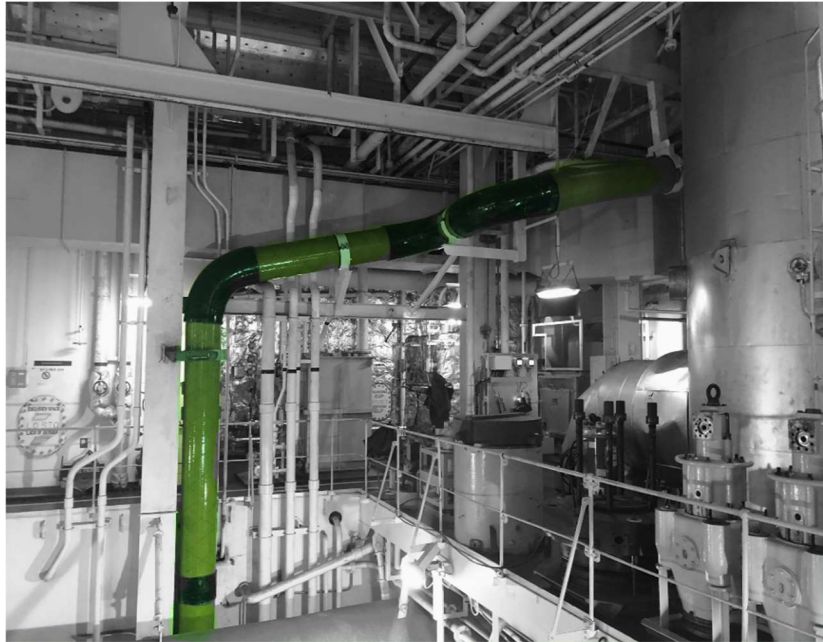
Scrubber washwater discharge GRE pipe fitted in an engine room
