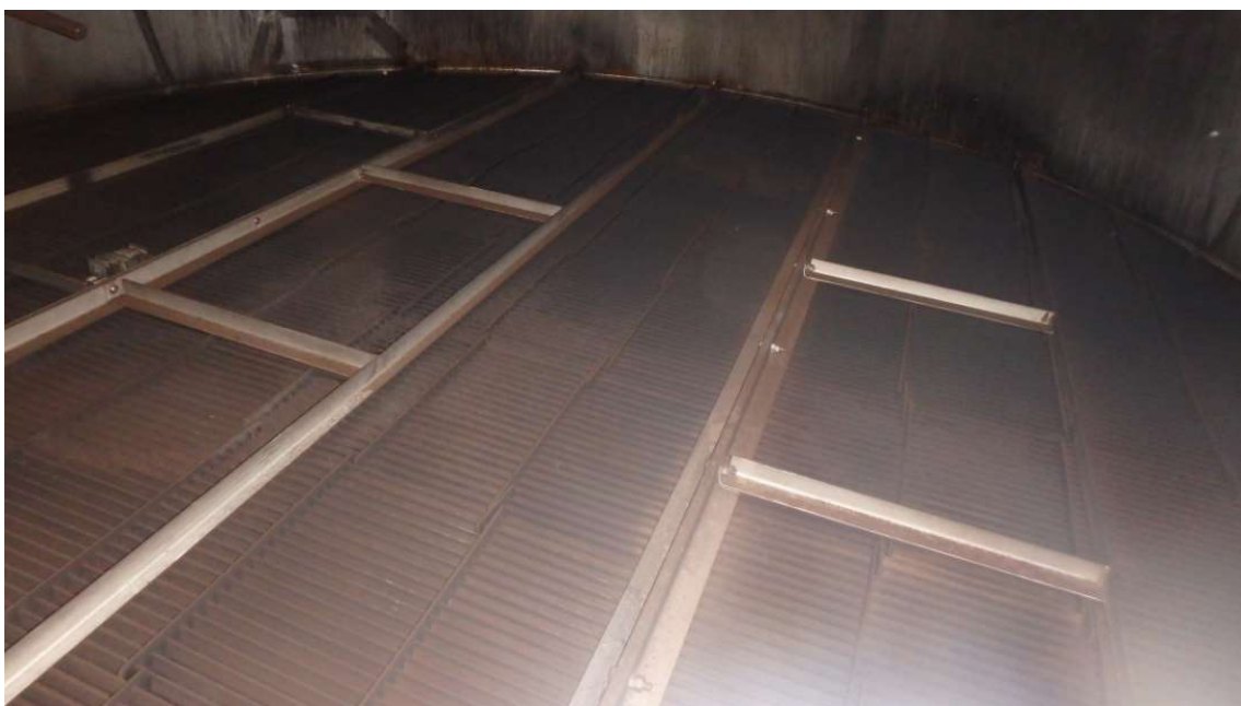
Demister section that is prone to soot build up when scrubber is run dry
