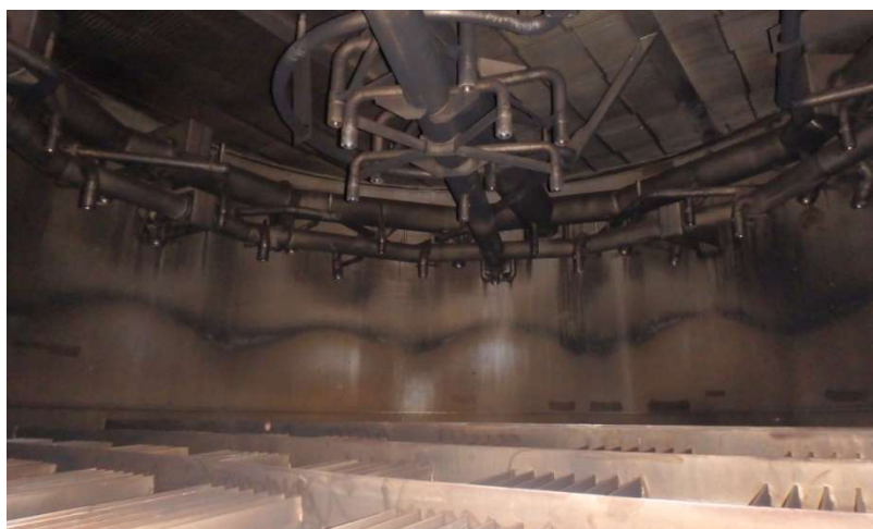
Interior of a scrubber tower with nozzles and demister
