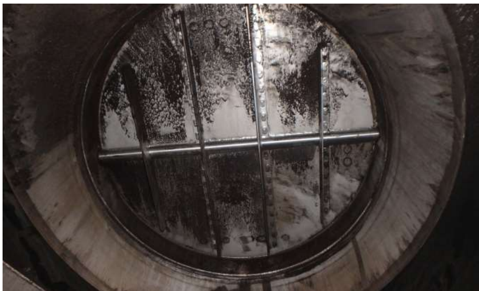
Interior of an exhaust gas bypass damper
