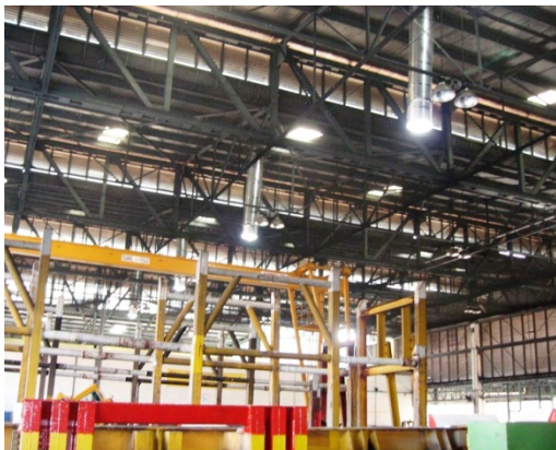
Natural day-lighting system in PSA Tanjong Pagar Workshop
